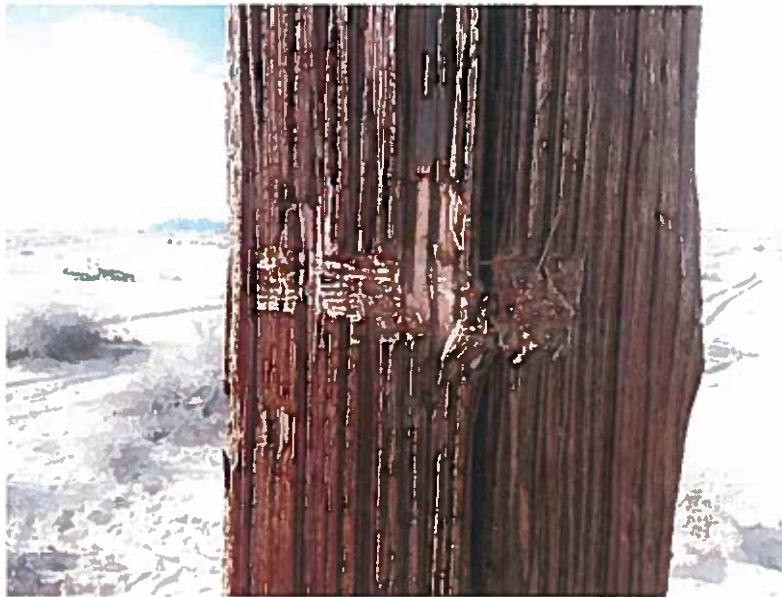
Figure 6: A scratch mark on Pole number 43502S.
