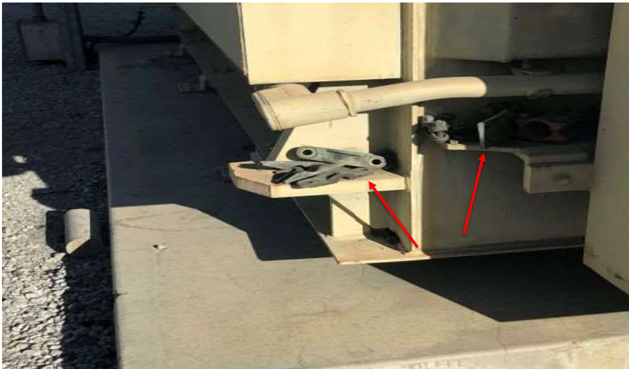
Figure 1: Parts left around Transformer Bank #2.
