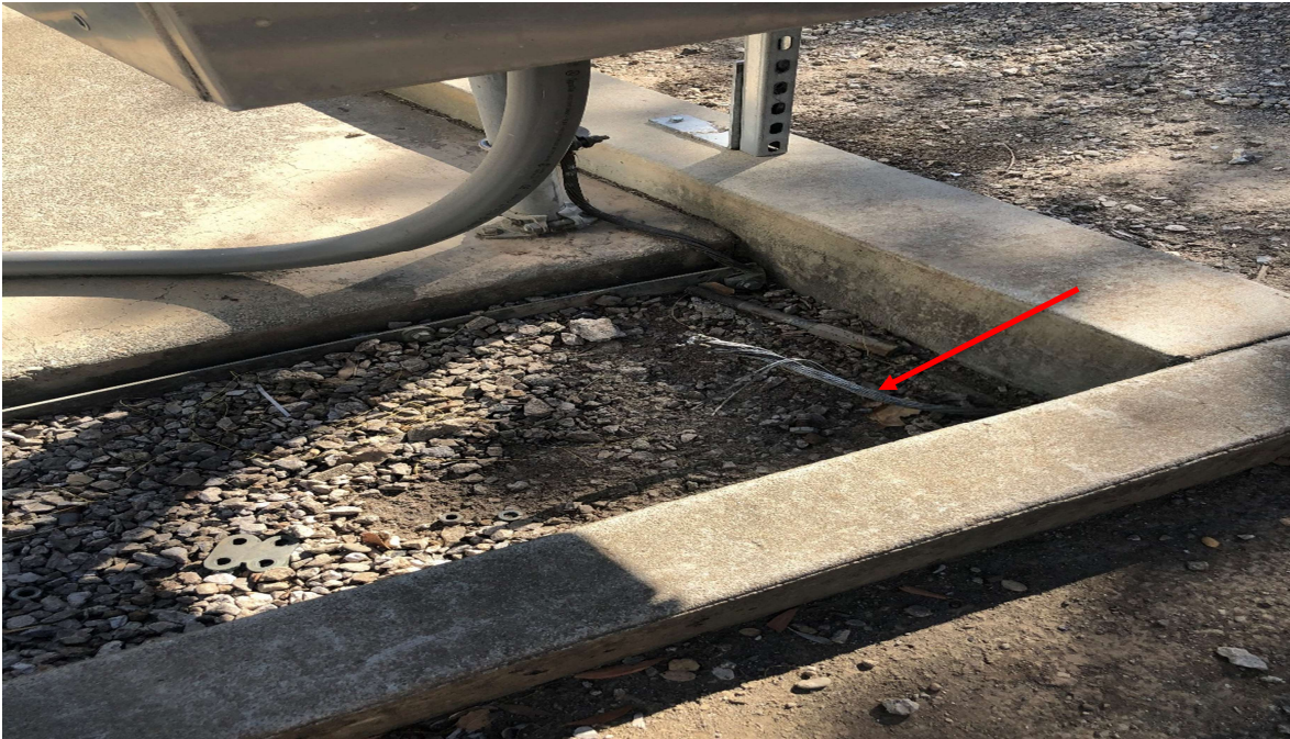
Figure 6: Abandoned ground wire protruding from the ground near Circuit Breaker #405.
