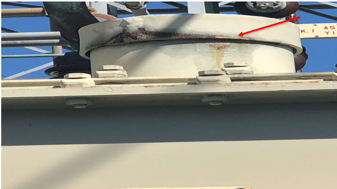
Figure 8: Potential oil leak on Regulator #403.
