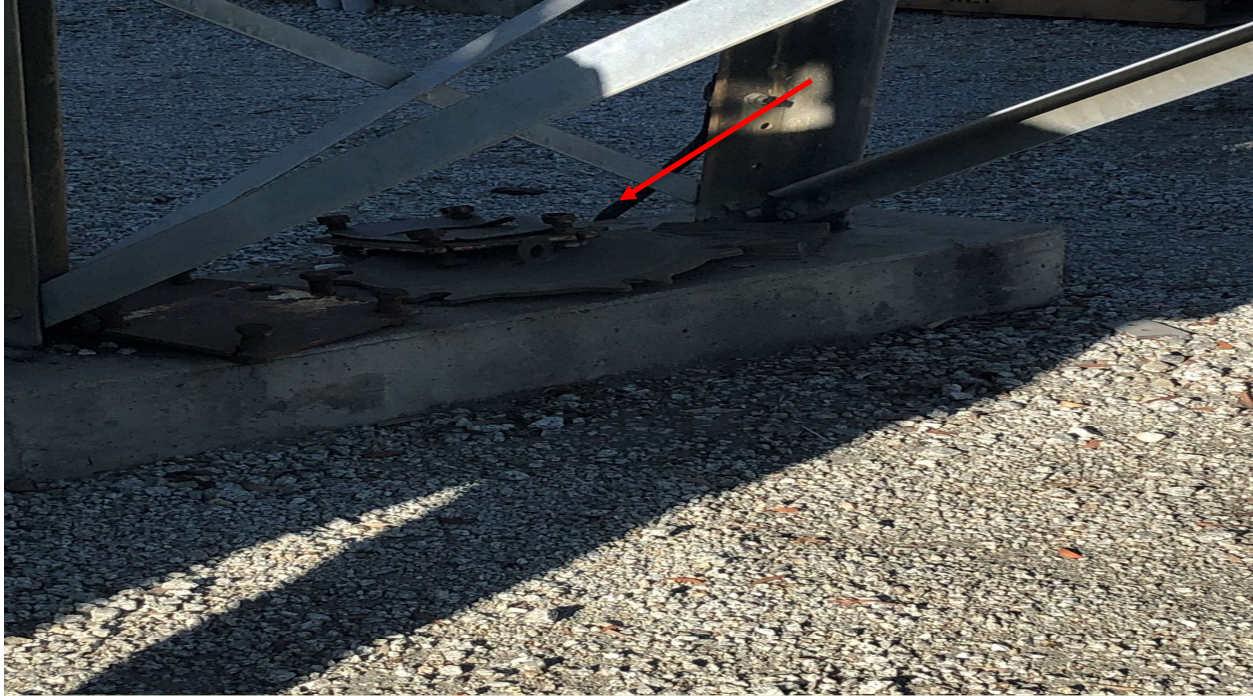
Figure 2: Parts left under Transformer Bank #2.
