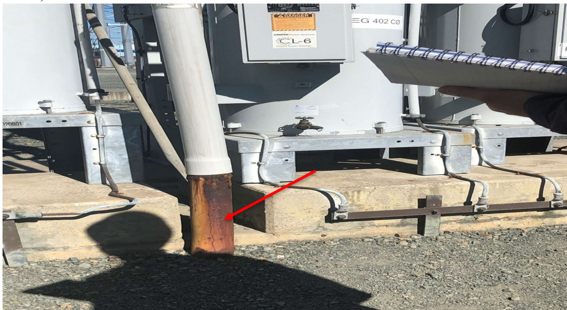
Figure 5: Atmospheric corrosion on the conduit supporting Regulator #401.
