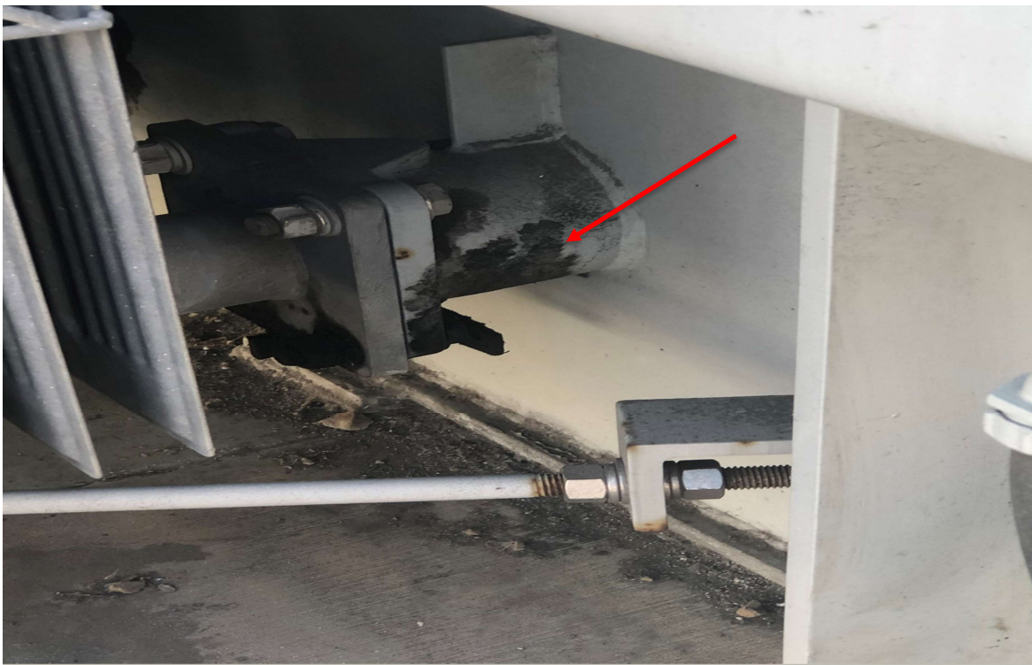
Figure 4: Example of oil weep at flange of one of the Transformer Banks.
