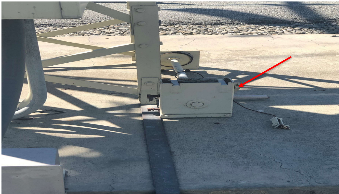
Figure 10: Lowering jack on the ground near Circuit Breaker #1101.
