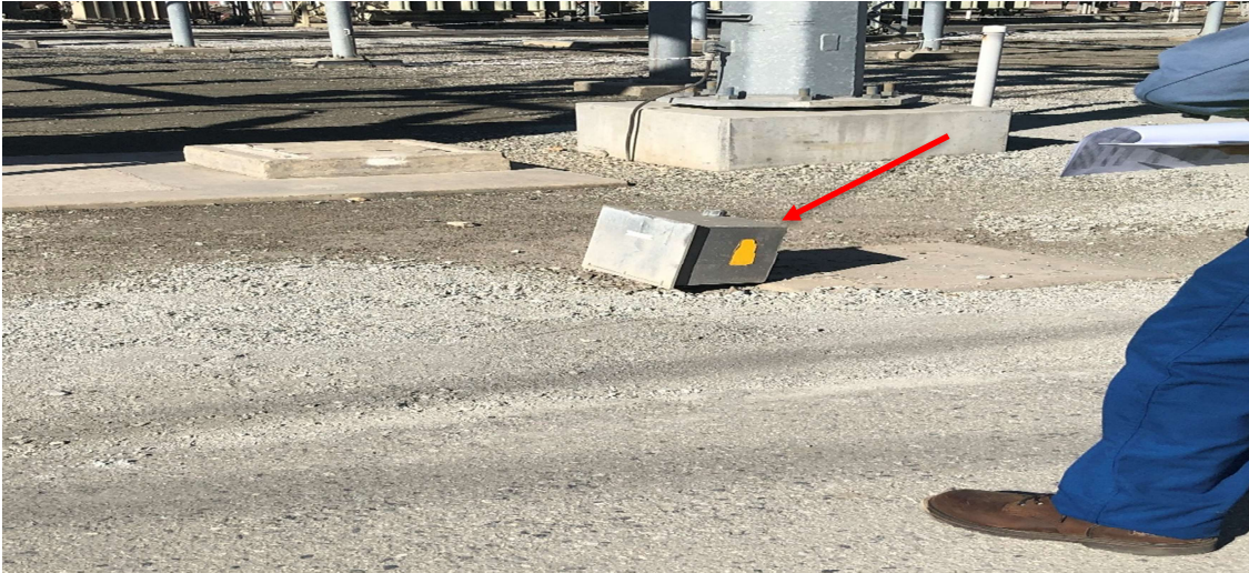
Figure 7: Junction box near Circuit Breaker #24.
