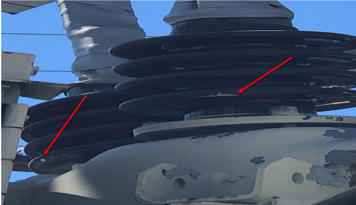
Figure 9: Chipped/ damaged insulator disk/bushing on Circuit Breaker #1101.
