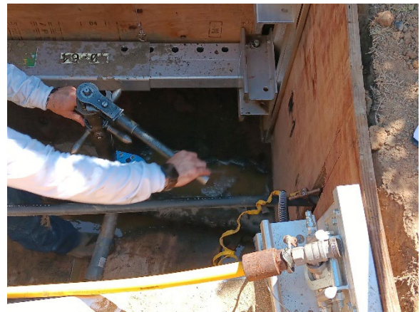
Connecting old and new pipe as part of mains and services replacement at a site in the Sacramento area
