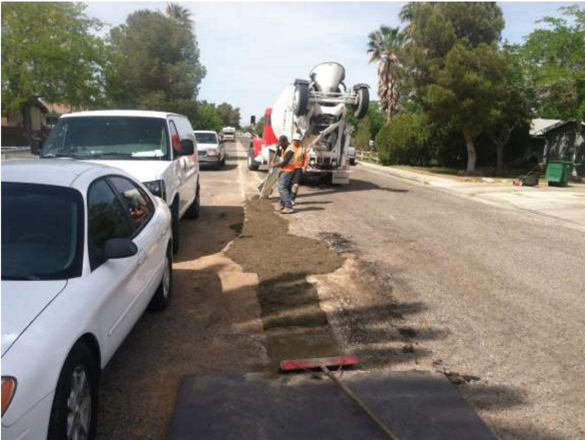
Figure 5 – Crews install a temporary patch over the trench for an underground telecom line along Lenore Street during the subject period. View north, 04/10/15.
