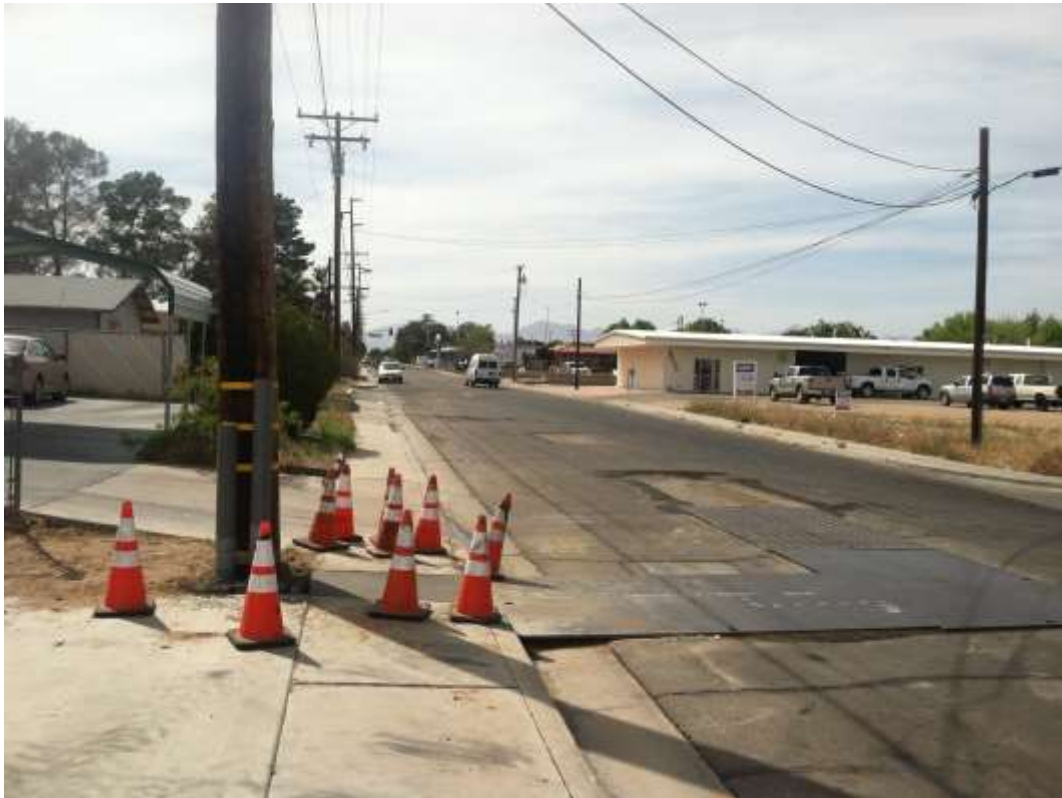
Figure 3 – Boring work for telecom lines continued during the subject period. The majority of underground work is complete. Steel plates are seen at the future location of the telecom line riser pole along East Church Avenue. View west, 04/10/15.
