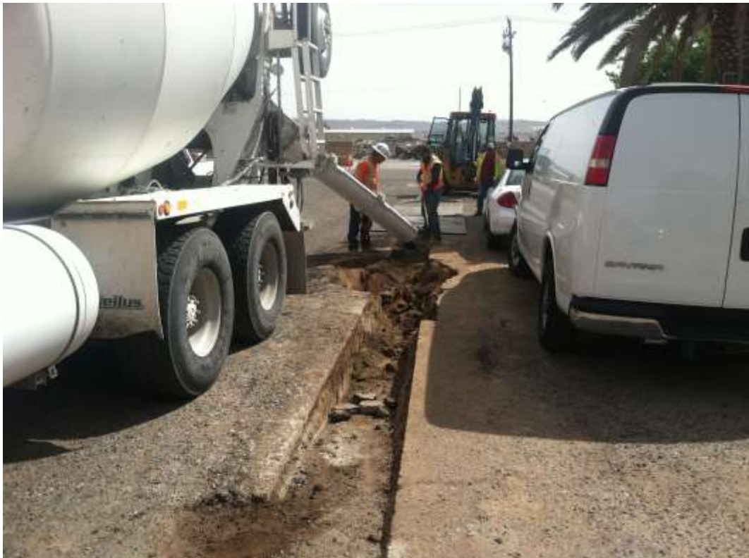
Figure 4 – Crews install a temporary patch over the trench for an underground telecom line along Lenore Street during the subject period. View south, 04/10/15.
