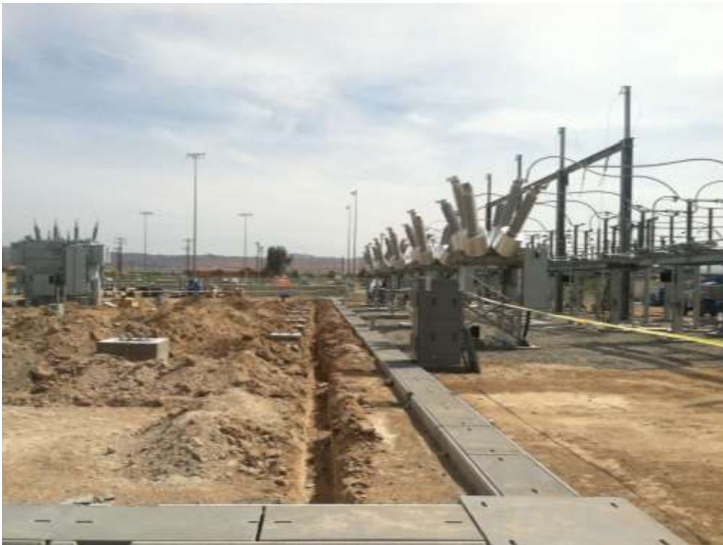
Figure 2 – Underground conduit installation occurred within the Substation expansion area during the subject period. View south, 04/10/15.
