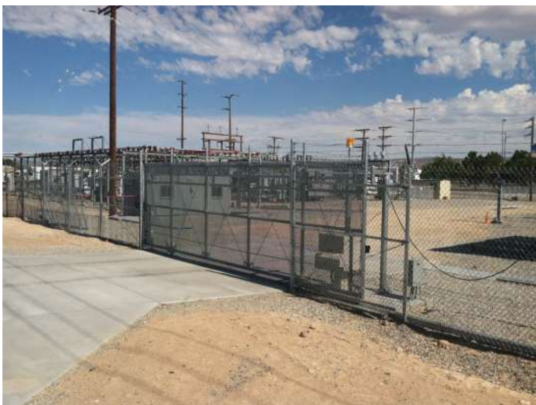
Figure 2 – Installation of a gate was completed during the subject period. View southeast, 6/24/15 above 7/1/15 below.
