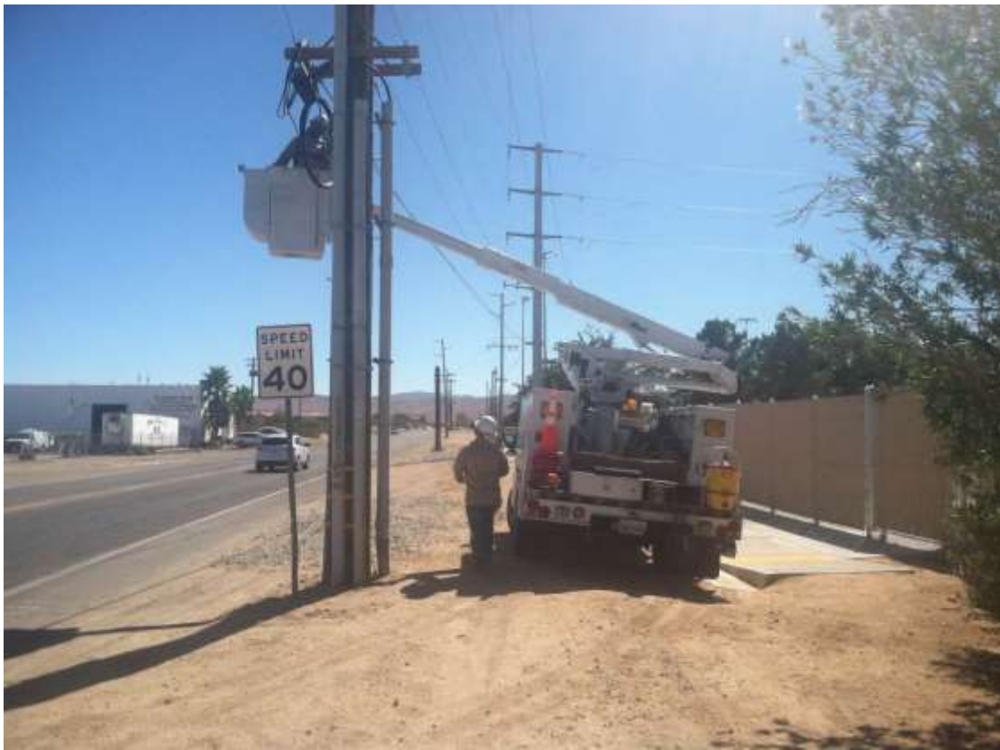
Figure 3 – Fiber line crews conducted some final checks during the subject period. Fiber optic installation was completed during the subject period. View south.
