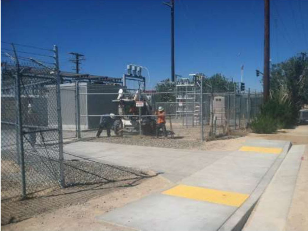
Figure 1 – Fence crews continued installing perimeter fencing at Downs Substation during the subject period. View northwest.
