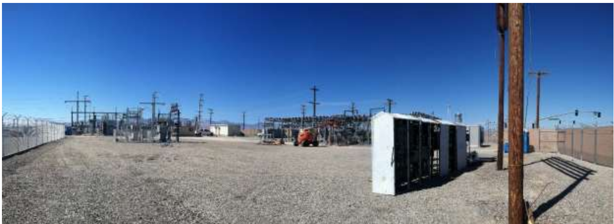
Figure 1 – Demolition work is largely complete in the old Downs Substation area. View northwest, 01/25/16 (top) 02/08/16 (middle) 03/17/16 (bottom).
