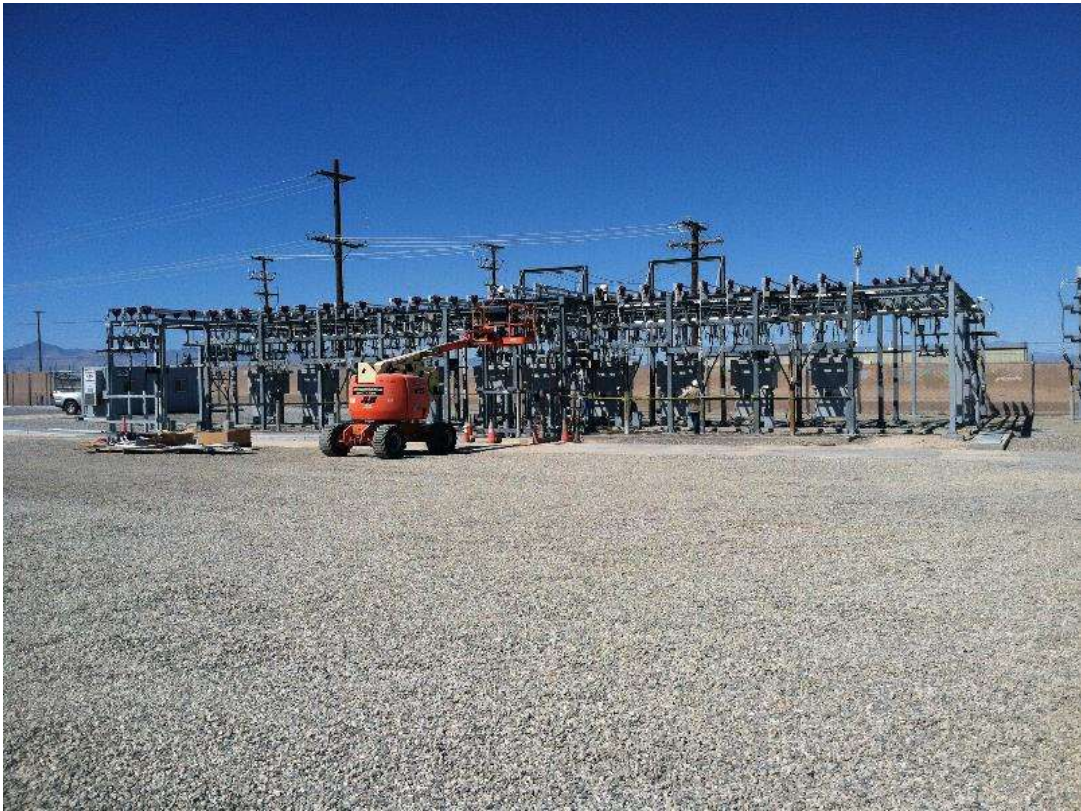
Figure 2 – Crews continued upgrading components of the old Downs Substation during the subject period. View northwest, 03/17/16.
