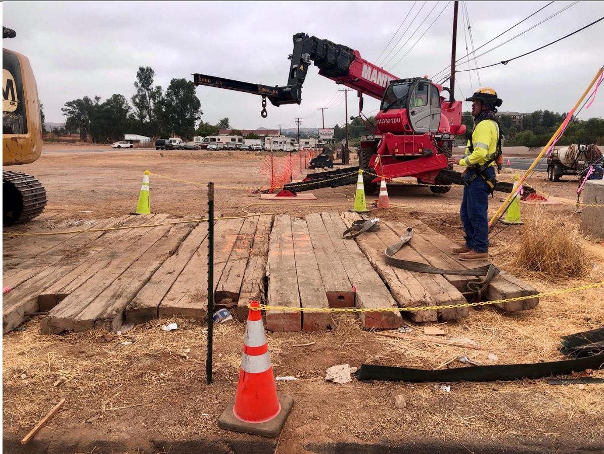
Photo 8 – The foundation hole had been drilled and covered overnight with wood planks. Photo facing east
