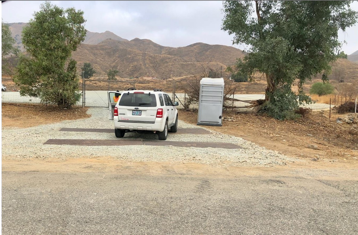
Photo 12 – Entrance to the Concordia yard with exit/entry BMPs installed. Photo facing east
