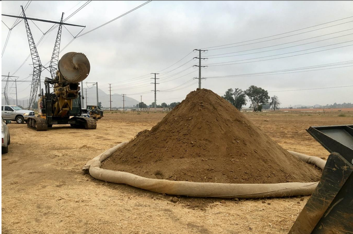
Photo 4 – The spoil pile from drilling the foundation hole at tower site #0018E. Photo facing north
