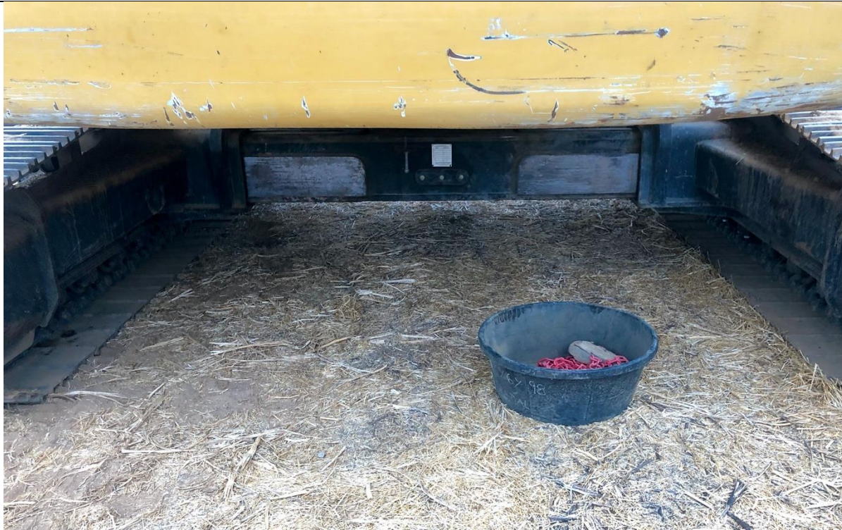
Photo 5 – Secondary containment under some equipment – note the small size of the drip pan and the material in it.
