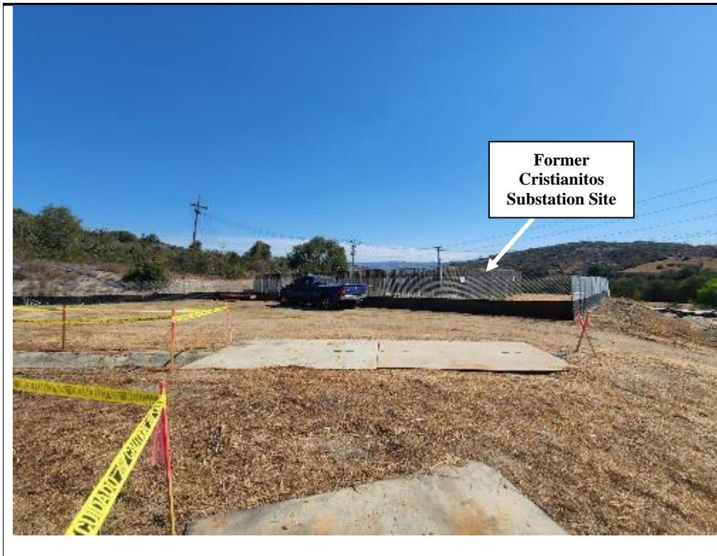
Photograph 5: View of the northwest corner of the Cristianitos Staging Area location with the former site of the decommissioned Cristianitos Substation shown. Facing: Northeast
