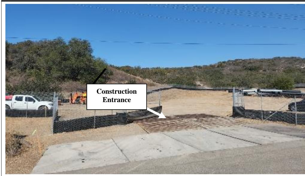
Photograph 1: View of the northeast corner of the Cristianitos Staging Area and northeast construction entrance. Facing: Southwest
