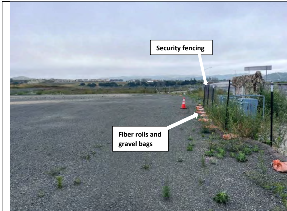
Photograph 2: View of Cow Camp Staging Area from construction entrance. The perimeter of the staging area contains security fencing and staked fiber rolls with gravel bags. Facing: East.
