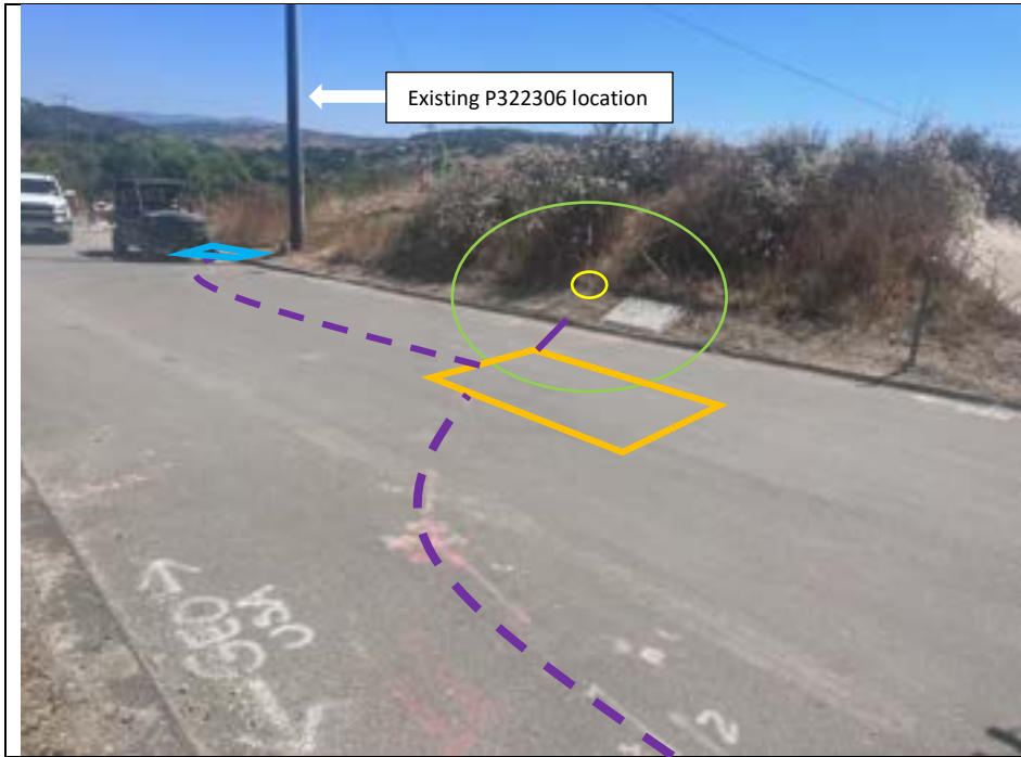
Photograph 4: View of the entire work scope involving trenching (indicated by purple dashing) from the Talega Substation to the new installed handhole (orange polygon) and then to the existing conduit located north of the existing P322306 location (blue polygon). Trenching will occur from the new handhole to the new P322306 location. Vegetation trimming will be required as needed within the CSS portion of the MPR-21 work area. Facing: Northeast.
