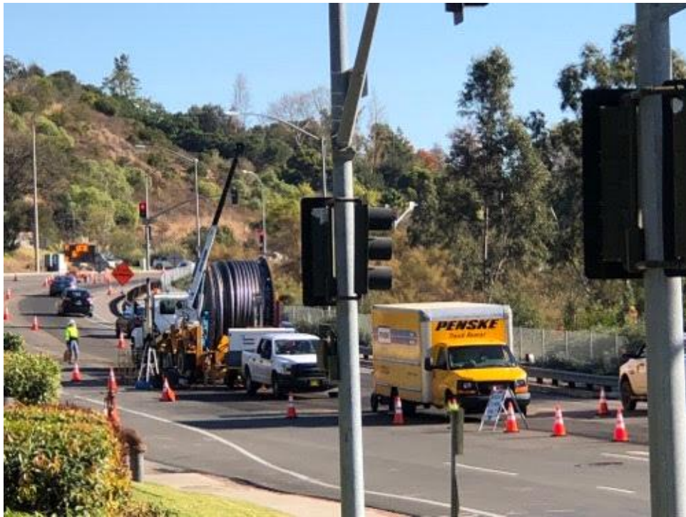
Cable install on Carroll Canyon Road just east of Nancy Ridge Road.
