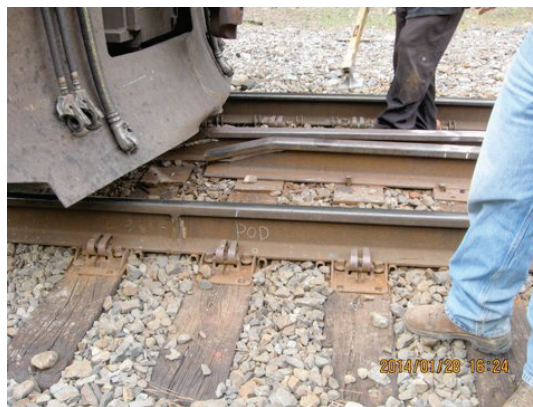
Point of derailment south of Gibson Siding at MP 301.8, at the entry to a railroad suspension bridge which spans the Sacramento River
