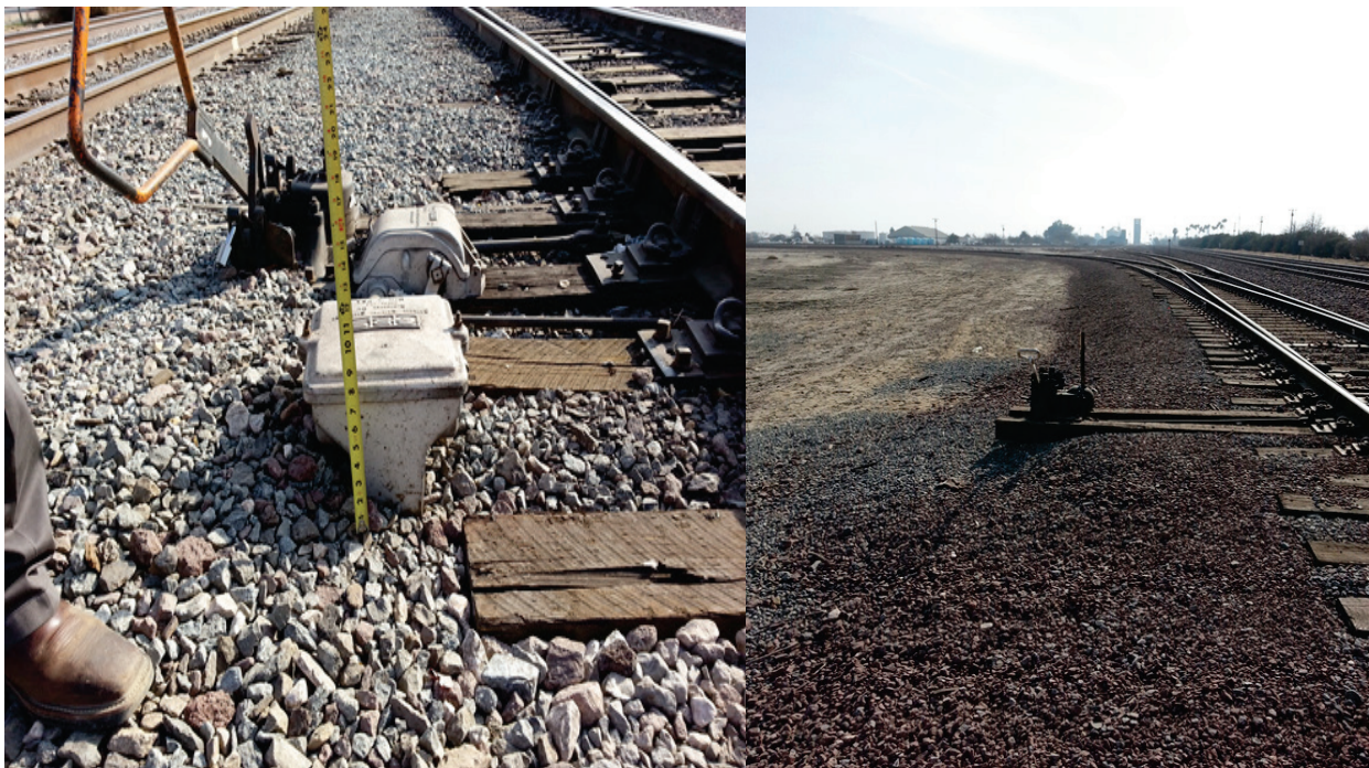
Photo to the left is a junction box that is in the walkway creating a tripping hazard for trainmen. The top of the box should be level with the walkway. Photo to the right shows a steep slope to the left of the switch. There is no safe place for a trainman to stand while lining the switch. A three foot level walkway is required behind the switch stand.
