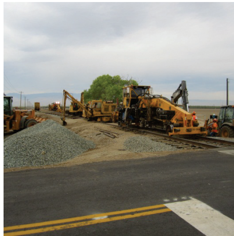
Rehabilitation along the Sunset Subdivision, southwest of Bakersfield, in preparation for crude oil train traffic.
