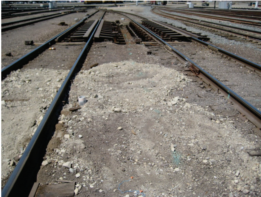
Rough and Uneven Walkway with Substantial Debris – GO 118 Defect UP West Colton Yard
