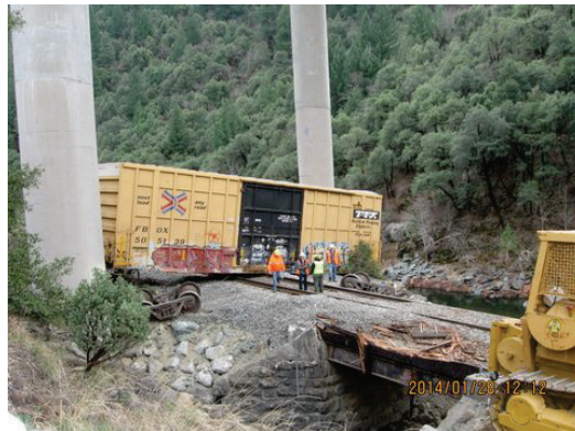
North end of Gibson derailment site, UPRR Milepost 304.23, just under I-5 Freeway Overpass at the confluence of Boulder creek/Sacramento River where one loaded and three empty boxcars left the rail.
