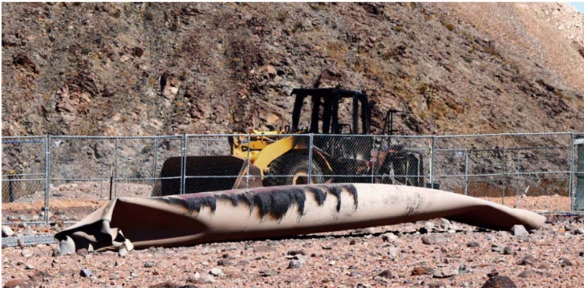
12 Figure 1-4: Ruptured Pipeline and Damaged 13 Equipment 105
